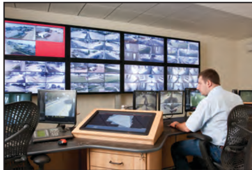
Control Room and Dispatch Center
